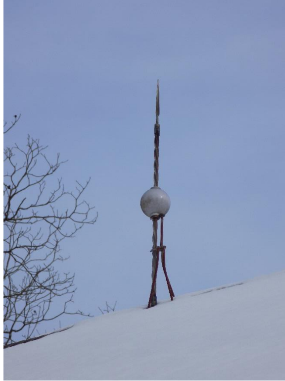
Lightning rod with glass ball located on top of Yost-Ketner home and log barn
